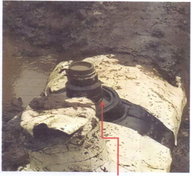
FIG.2 Incident facility after exposure 6" inch valve
